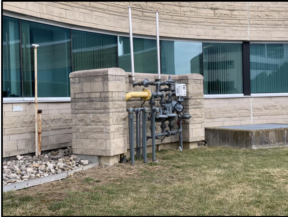
Image 15: Sympathetically designed gas metre housing (Photo taken on March 11, 2020; Facing North)
