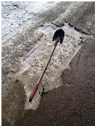
Example of core assets with condition defects: winter freeze and thaw damage.
