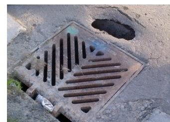
Example of core assets with condition defects: drainage damage caused by a broken pipe.
